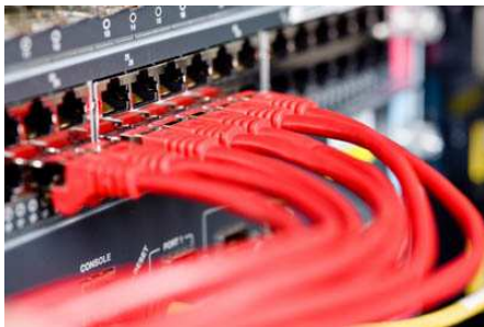
Caption: Siemens IT Solutions and Services will implement green and sustainable modernization on around 25,000 servers throughout Germany in the coming years. In a few data centers, such as Fürth or Munich, blade servers are already operating together with an energy-saving cooling system. (Source: Siemens)
